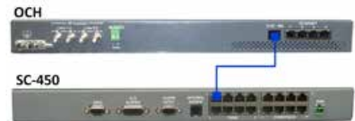
Figure 5. OCH-to-SC-450 Management Connection
