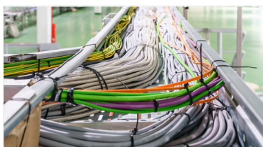
Legacy Category Cable Network
