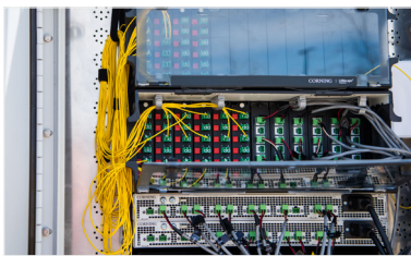
Consolidated power distribution at a single location
