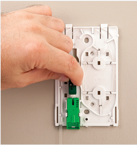
Connecting 900 µm Fiber Pathway Inside Low-Profile Wall Plate
