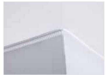
Clear Track Hallway Fiber Pathway Installed Around Exterior Corner
