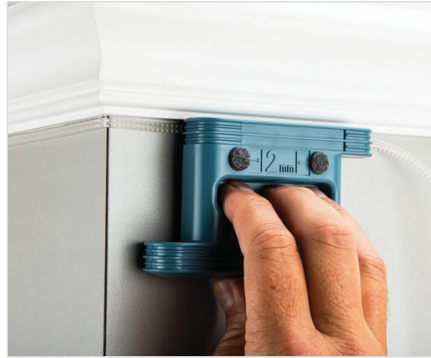
Installation of Hallway Fiber Pathway with Clear Track Hallway Universal Installation Tool
