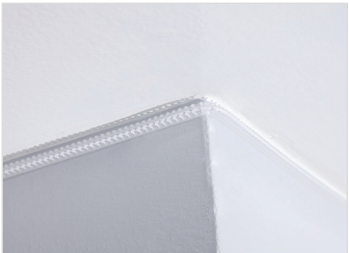
Clear Track Hallway Fiber Pathway Installed Around Exterior Corner
