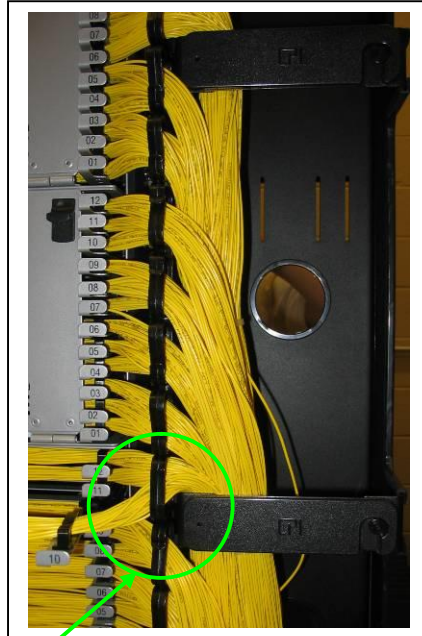
Pinch points and sharp edges
