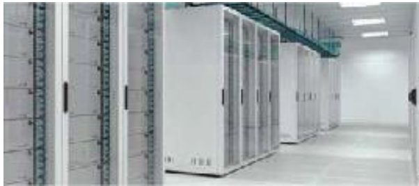
Data centres use advanced optical cabling solutions
