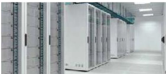
Data centres use advanced optical cabling solutions
