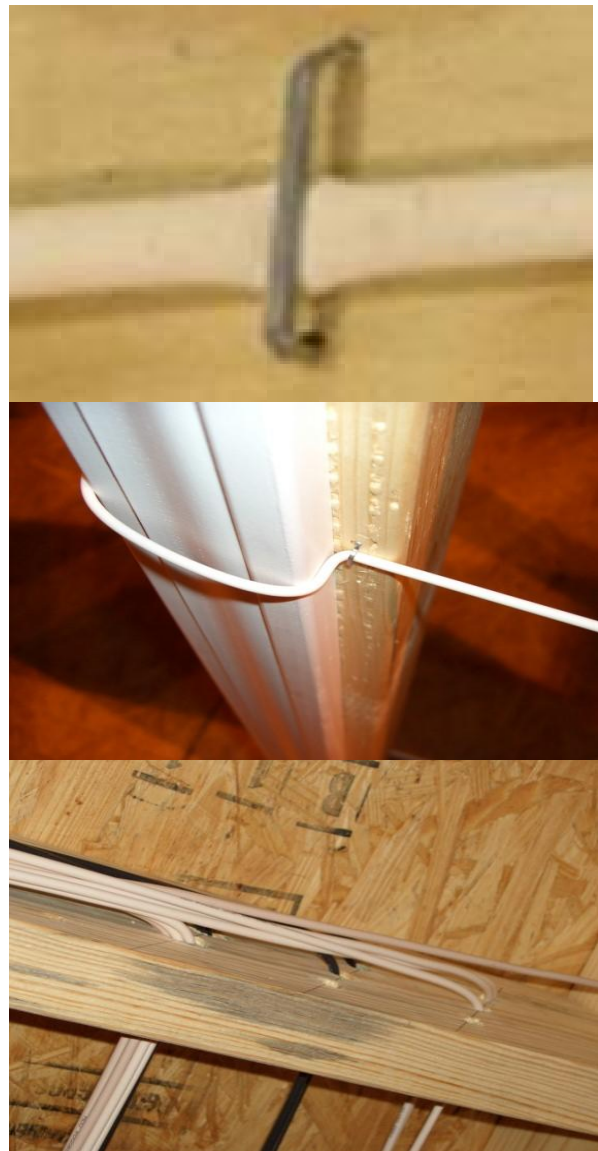
Fig. 1: Examples of in-building cable installations; stapling and cornering
