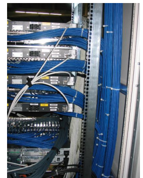
LANscape Modular Patch Panels & Copper Cabling
