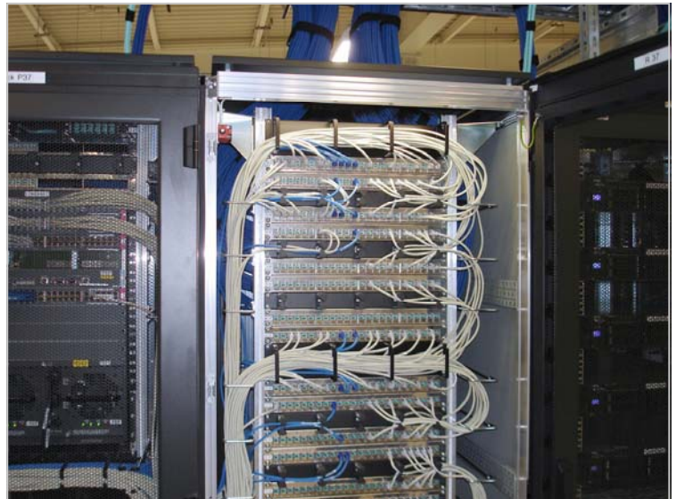
10 Gigabit Shielded Copper Cabling in the Ernst & Young Data Centre
